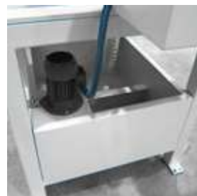
__ tank and water pump: cooling system in a closed circuit
